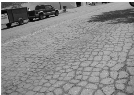
Figure 1 Example of fatigue cracking occurring on the HMA pavement
