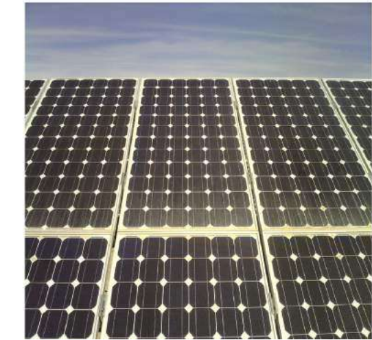
Figure 16 Overheated module with a \Delta T of 10.5°C between the mean temperature of the adjacent modules and the mean temperature of the overheated module surrounded in the figure
