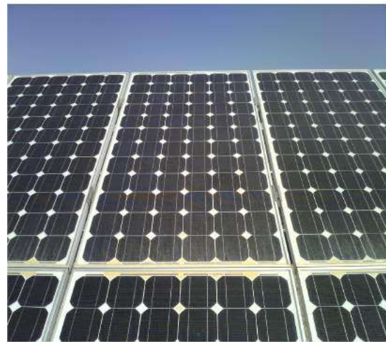
Figure 4 Hotspot located in the third string of a module, with a \Delta T of 71^\circ\text{C}
