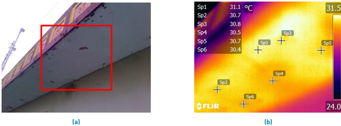
Figure 13 Lower area of the Maurício de Nassau Bridge sidewalk: a) Digital image and b) Thermogram. Source: The Authors
