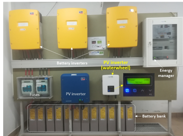
Figure 12 Smart microgrid installed in Castrelos' Aquaculture Centre
